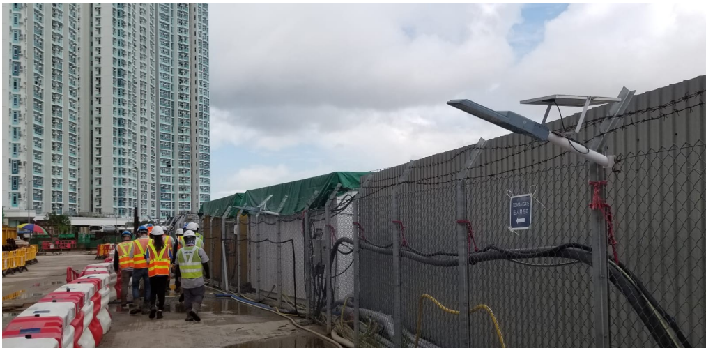
Photo 5 – Orientation of night time lighting to minimize glare impact
